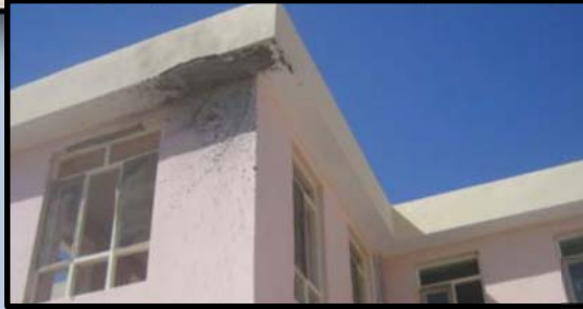
Damage from rocket propelled grenades.
